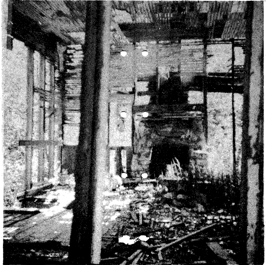
INTERIOR of what's left of the ranch house where Stevenson nearly died.
